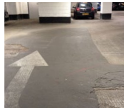
POOR QUALITY REPAIRS
