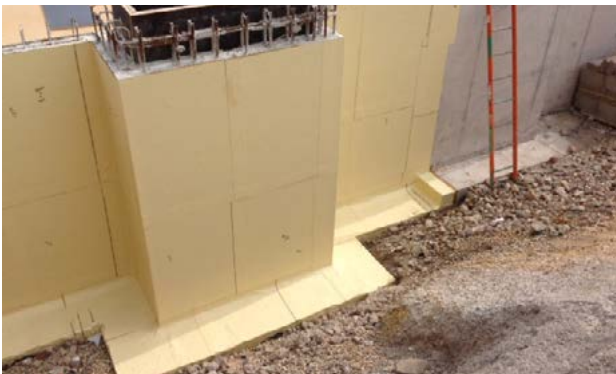
Open excavation with protrusion slab to wall: The complete structure is sealed with SikaProof® P.
