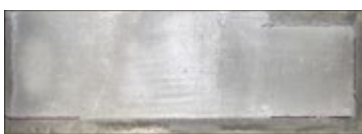
Mortar with good crack behavior.
