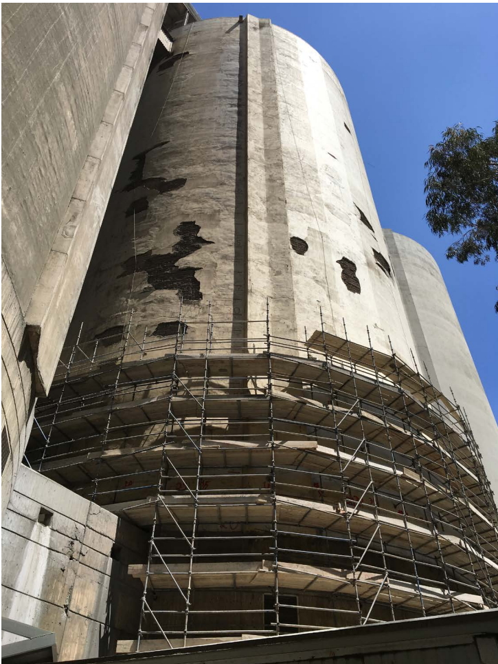
Before remedial works.
