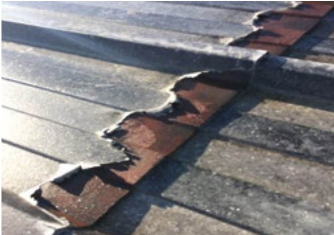
Corroded roof sheet
